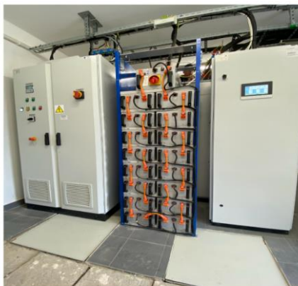
LTO based energy storage inside transformer station
