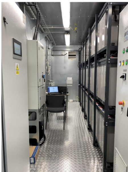
VRLA based energy storage inside sea container
