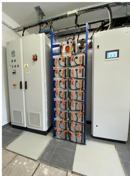
LTO based energy storage inside transformer station
